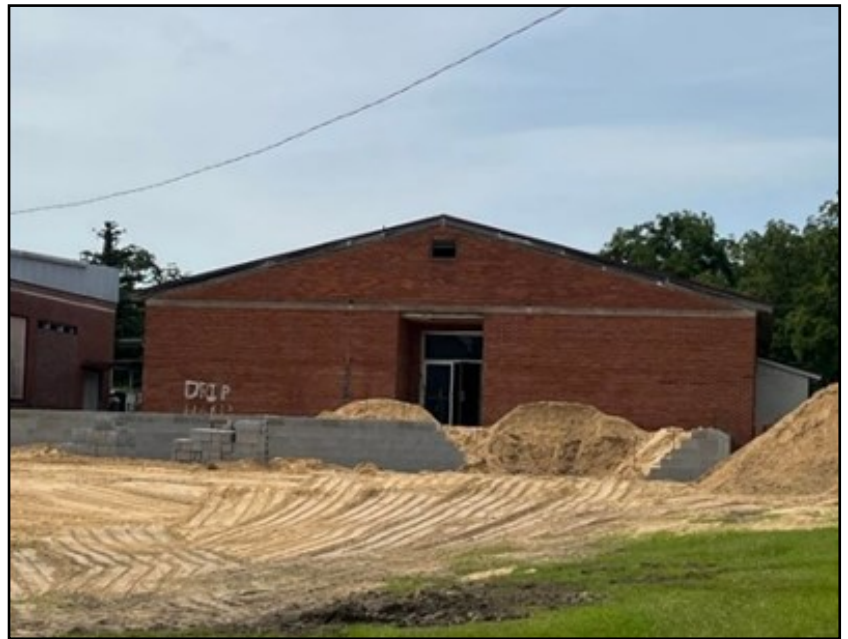
Construction work to expand the Monitor Enrichment Center in Ben Hill County
